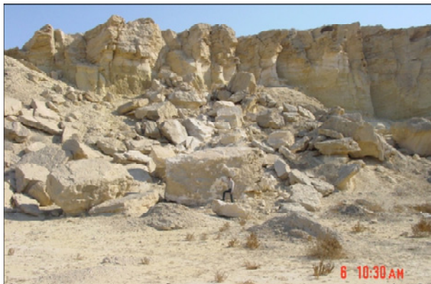
Figure 6. Wide crack tensions along the cliff edge of wave-built terraces formed in upper hard layer.
