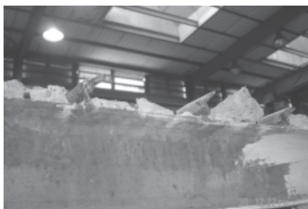
b) Shearkeys Action after Failure of the Slab Concrete
