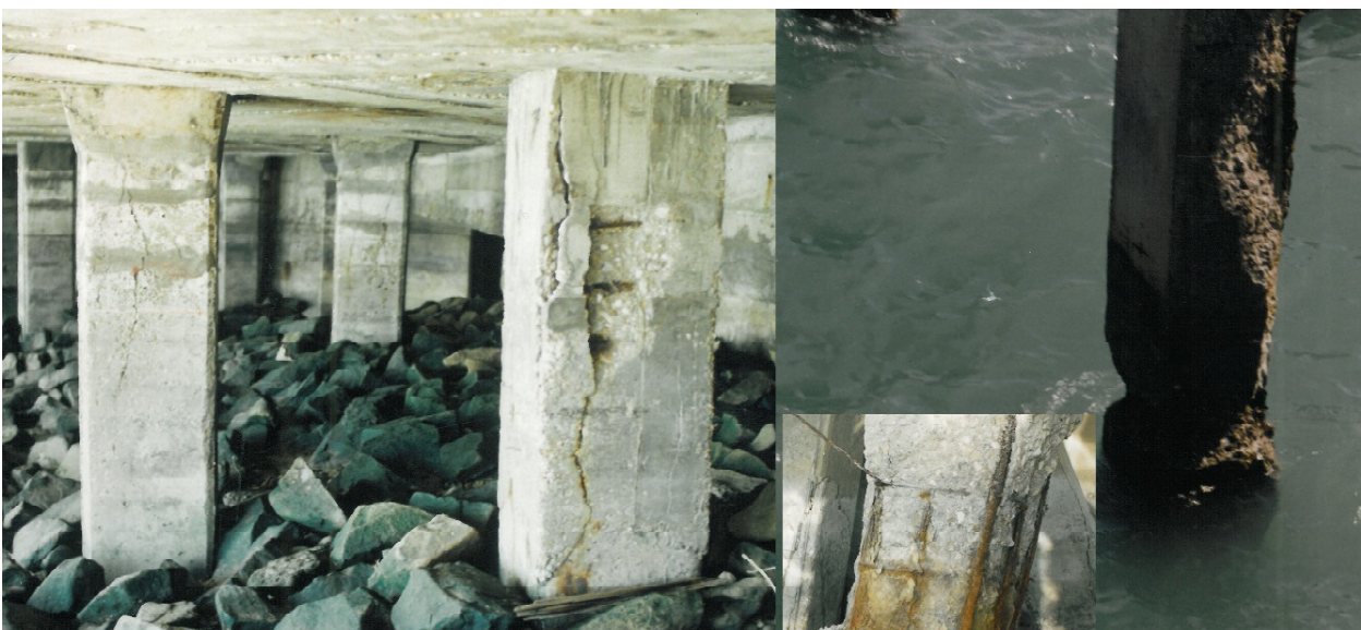
Figure 1. Examples of corroded RC piers exposed to seawater in Persian Gulf zone, Boushehr
