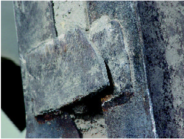
Figure13. Rupture of battens in a pharmacy.
