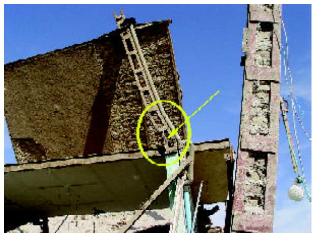
Figure 10. Local buckling of one chord of batten column.
