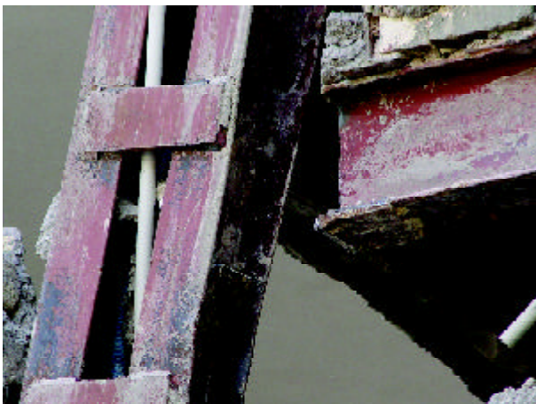
Figure 6. Rupture of seat angle of simple connection.
