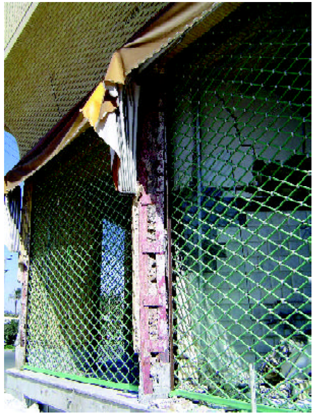
Figure 9. Overall buckling of batten columns about hollow axis in a store.
