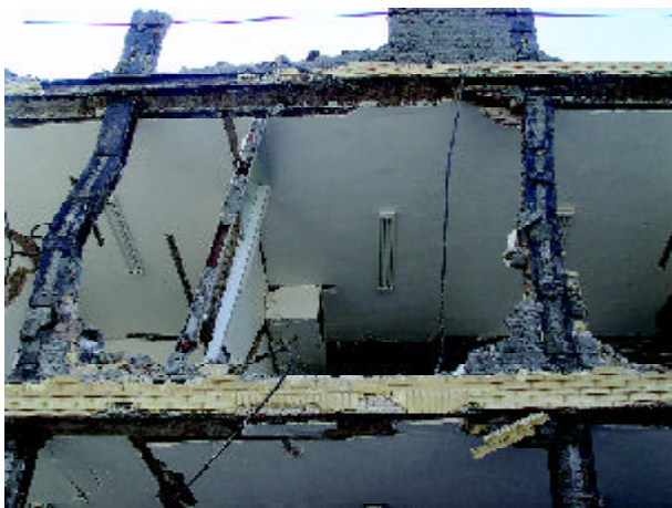
Figure 8. Overall buckling of batten columns about hollow axis in a pharmacy.
