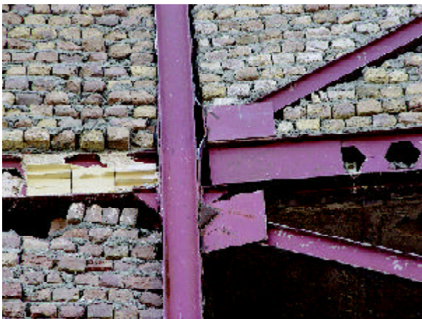
Figure 7. Separation of connection plate of batten column.
