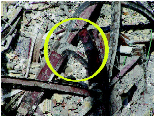
Figure19. Failure of batten column in splice location in kimia building.
