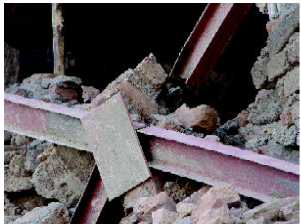
Figure 3. Rupture of connections in concentrically X bracing.
