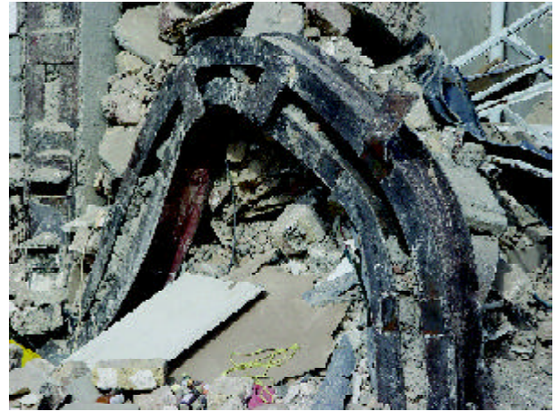
Figure 16. Weld rupture in all battens of batten column in a pharmacy
