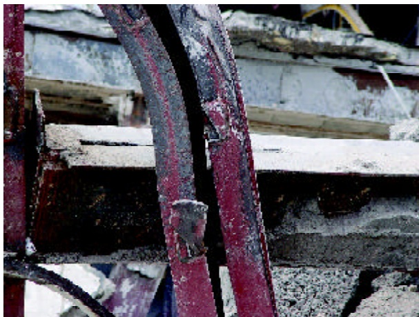
Figure 14. Rupture of battens in a shopping center.
