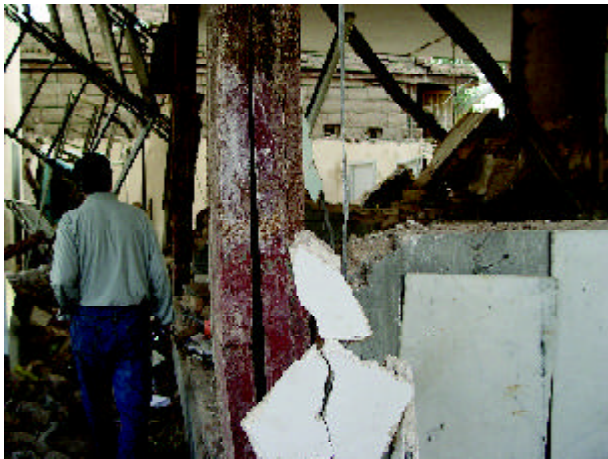
Figure 1. Rupture of longitudinal joint in box column.
