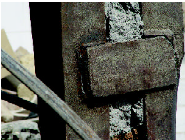
Figure15. Weld rupture in battens of batten column in a pharmacy.
