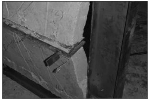
Figure 9. Out of plane deformation of EIF-0.5.
