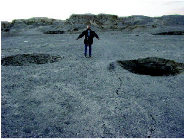
Figure 18. Collapse of shafts and tension crack along the galleries of old Qanats, west of Baravat.
