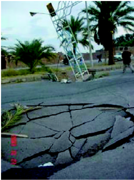
Figure 22. Damages to road and a religious arc due to the collapse of a hidden Qanat (Baravat). Photo has been Taken by Dr. M. Zare one day after the event.
