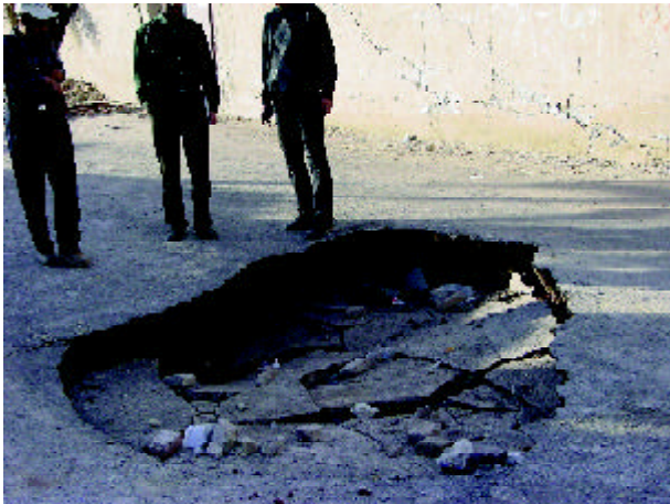
Figure 19. Sinkhole induced due to collapse of an old Qanat on one of the bypasses at Baravat.
