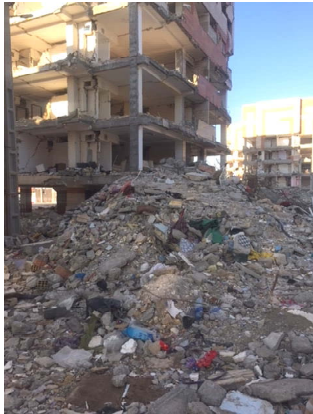
Figure 1. Damage to residential complexes (photo: Izadkhah).
