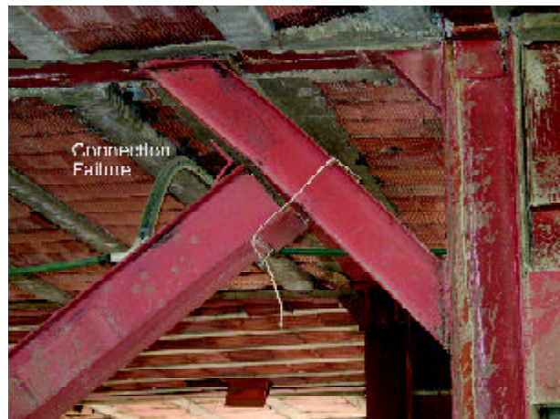
Figure 18. Failure of bracing connections to frame.
