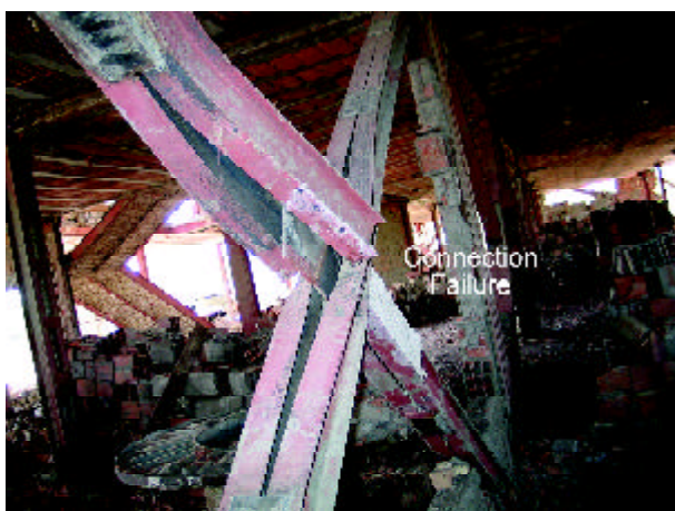
Figure 16. Failure of cross bracing connections.
