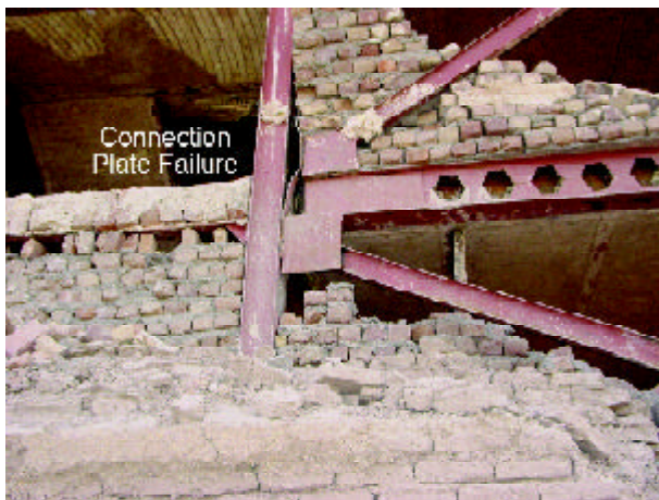
Figure 14. Fracture of bracing-to-frame connections.
