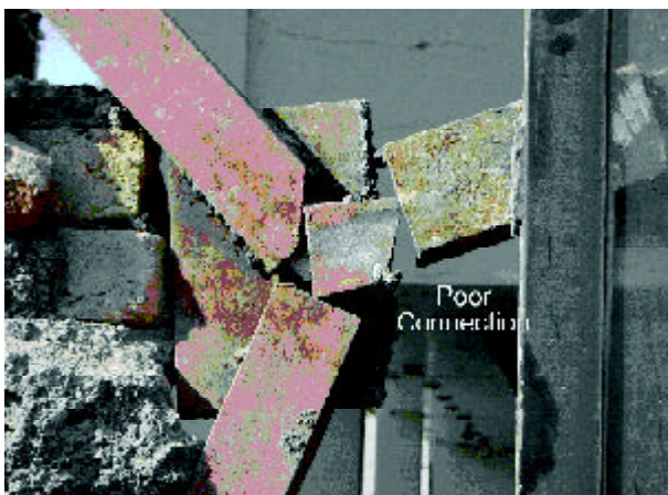
Figure 21. Very poor bracing connections.
