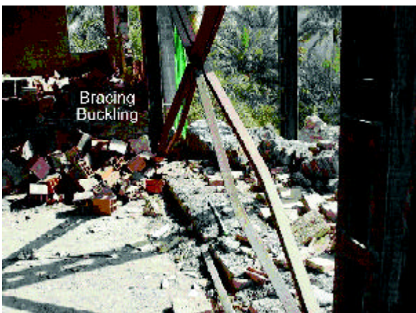
Figure 26. Out of plane buckling of built up bracing.
