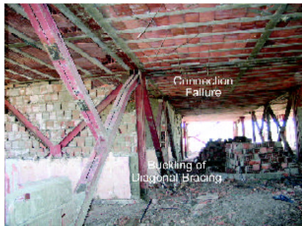
Figure 17. Buckling of diagonal bracings.
