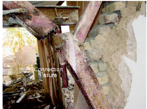
Figure 22. Fracture of bracing connections.
