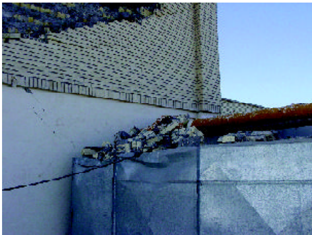
Figure 25. Damage to air conditioners.
