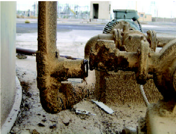
Figure 19. Rupture of pipe connections.
