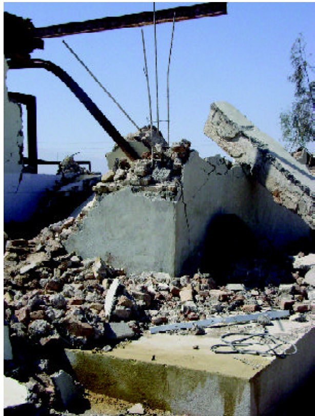
Figure 7. Collapse of chlorination building.
