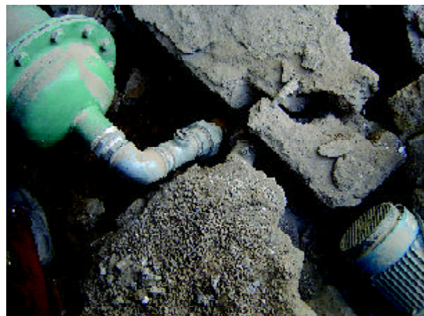
Figure 15. Damage to equipment in the collapse of mechanical buildings [1].
