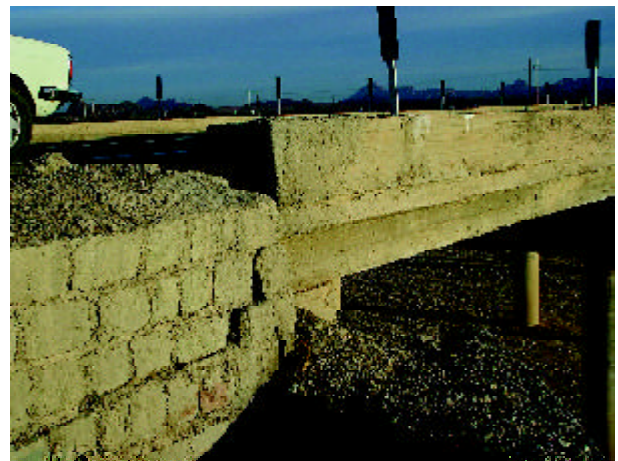
Figure 12. Settlement of Darzin bridge abutment.
