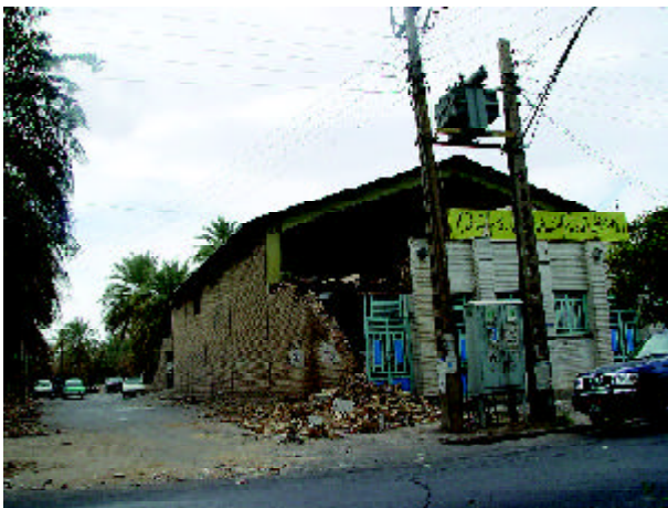
Figure 13. Damage to annex building of an industrial frame [1].
