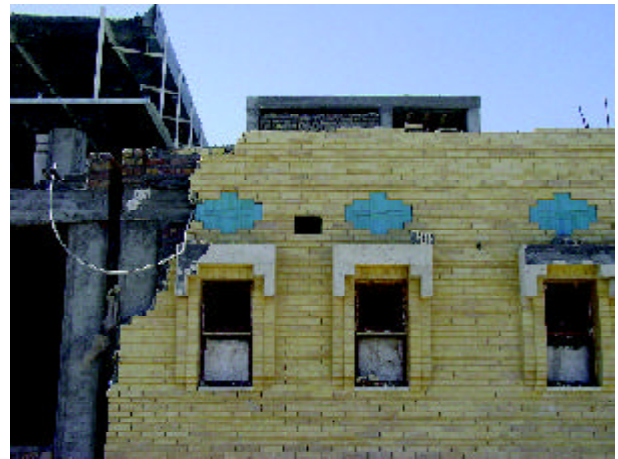
Figure 26. Damage to façade at the Bam train station.
