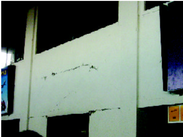
Figure 24. Damage to masonry infill walls at airport.
