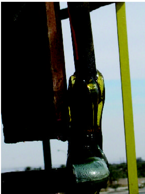
Figure 21. Leakage of oil due to rupture of pipes [1].
