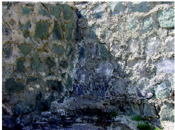
Figure 8. Leakage of water from tank wall.
