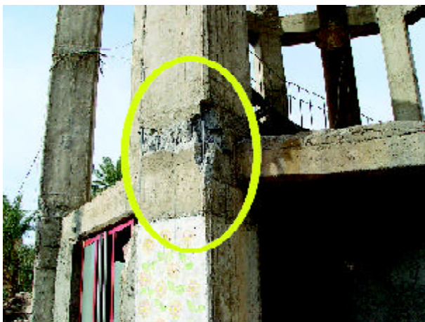
Figure 4. Inaccurately detailed cracked RC column [1].
