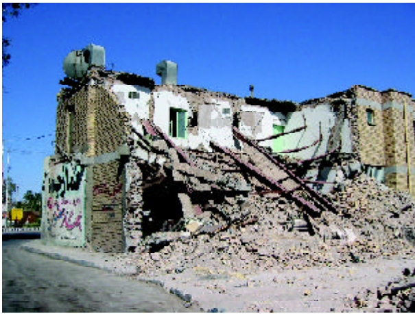
Photo 2. Collapse at the south west section.
