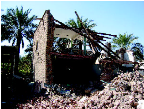
Photo 6. Collapsed two-story school building.
