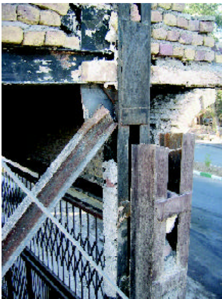
Photo 8. Fracture of welded joint of a steel brace.
