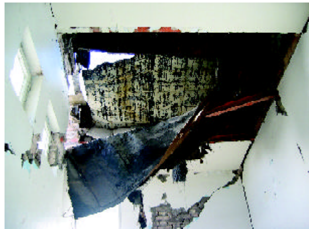
Photo 4. Falling down of the roof of penthouse.
