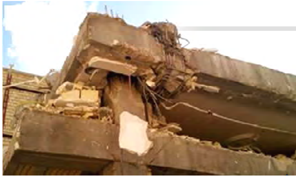
Figure 18. Punching shear in an RC structure during the 12 th November 2017 earthquake.
