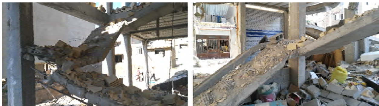
Figure 14. Staircases separated the structures by the brace performance due to poor implementations.
