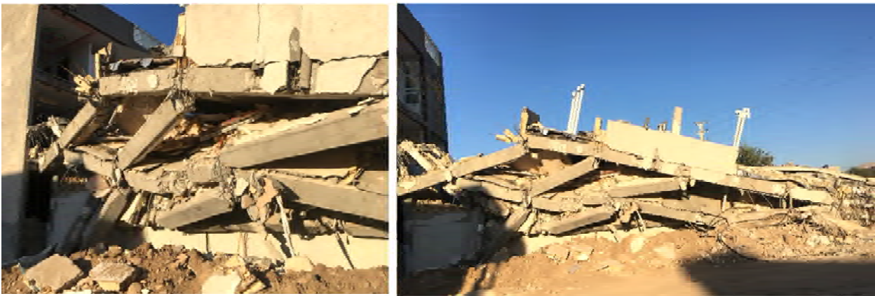
Figure 12. The pancake collapse of structures under Sarpol-e Zahab earthquake.
