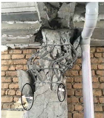
(e) Column Failure with Buckled Longitudinal Bar and the Unequal Cover at the Slides of the Column
