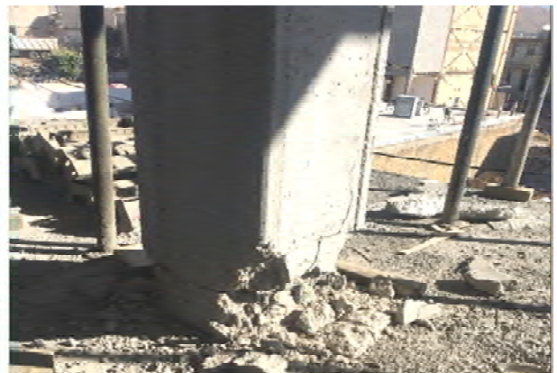
(b) Loss of Concrete Cover That Caused by Flexural Damage
