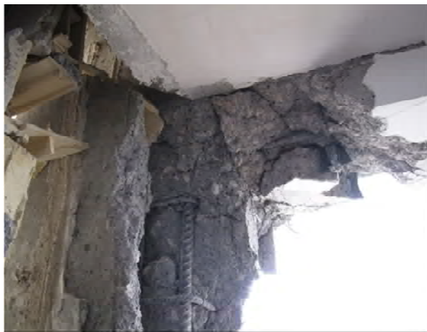
Figure 31. Failure at the bottom flange of a beam with slab.
