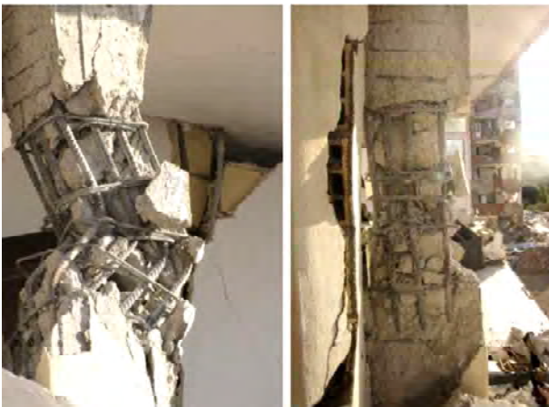
Figure 5. Sample of structural Damage in Sarpol-e Zahab, and Shahid Shiroudi Mehr buildings.
