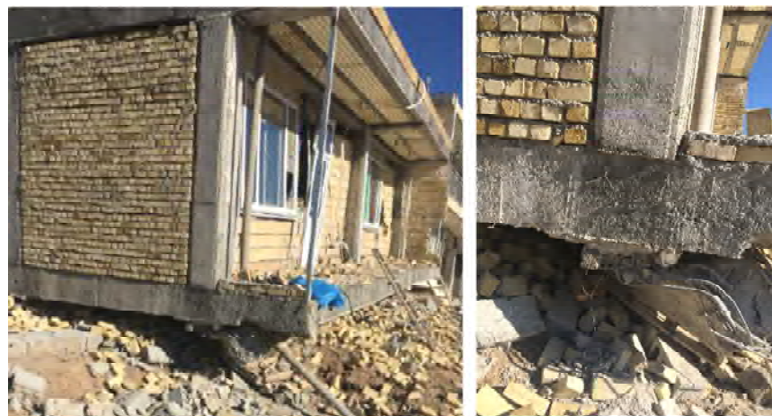
Figure 13. The torsional collapse of the structures subjected to Sarpol-e Zahab earthquake.
