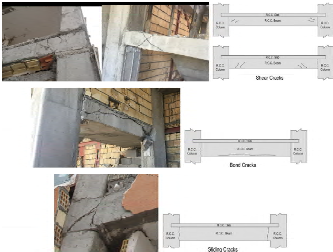
Figure 32. Damage patterns of RC beams under Sarpol-e Zahab earthquake [37].
