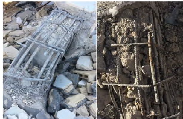
Figure 21. Imperfections in implementation of transverse reinforcements, Eslamabad-e Gharb hospital.
