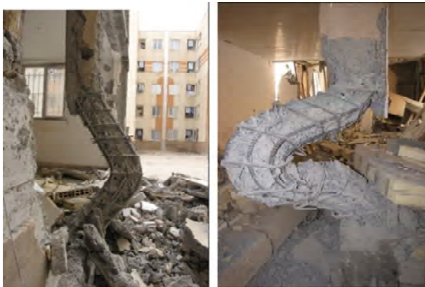
Figure 33. Buckling of structural columns in Eslamabad-e Gharb, Mehr buildings.
