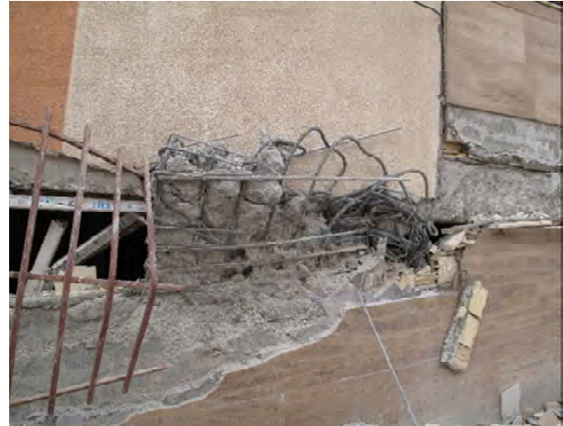
Figure 38. The failure of shear wall because of inadequate anchorage of longitude reinforcements in Eslamabad-e Gharb, Mehr buildings.
