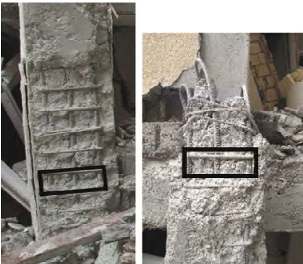
Figure 27. Imperfections in transverse reinforcements spacing in Eslamabad-e Gharb, Mehr buildings.
