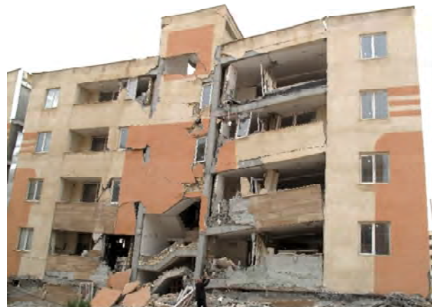
Figure 8. Earthquake damages caused by weak-story in Eslamabad Mehr buildings.
