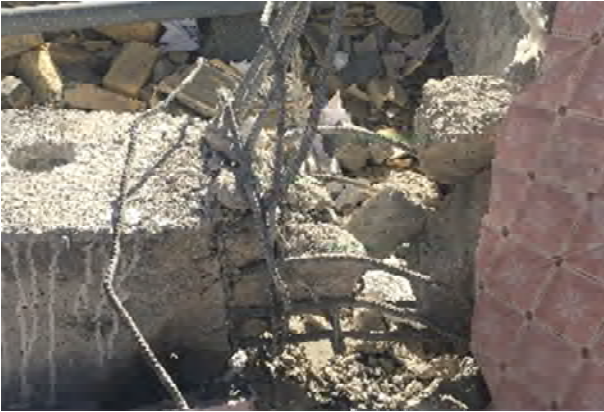
Figure 26. Sliding the bars in concrete due to the low quality of materials.
