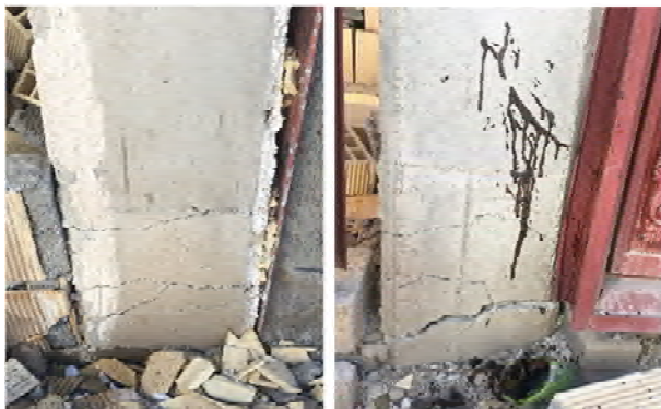
(c) Visible Horizontal Cracks That Caused by Flexural Damage
