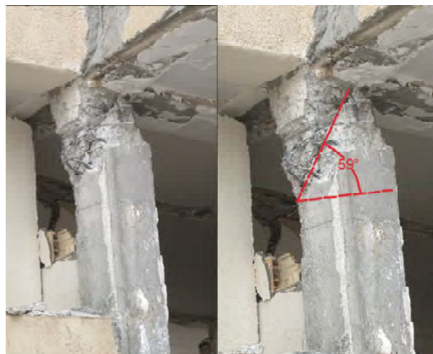
Figure 22. Shear failure, Eslamabad-e Gharb Mehr building.
