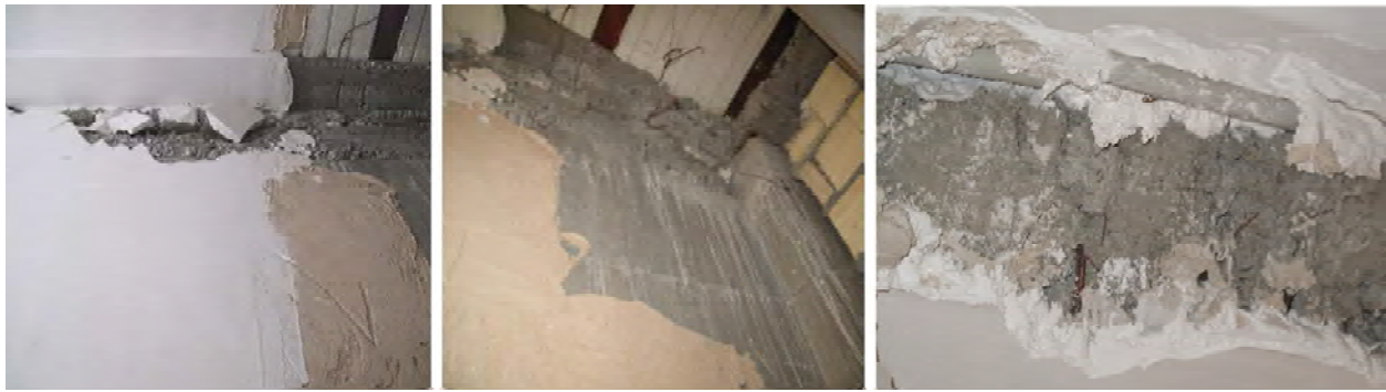
Figure 36. The low quality of concrete used in Eslamabad-e Gharb, Mehr buildings.
