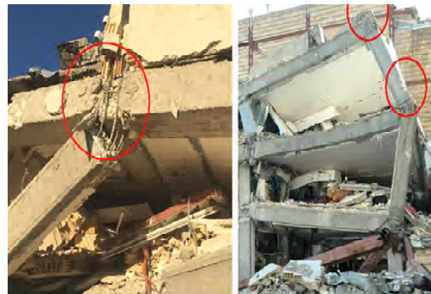
Figure 24. The shear failures due to the lack of ductility in joints.
