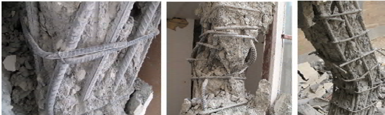
Figure 30. Imperfection in using 135 degree hooks in transverse reinforcements.
