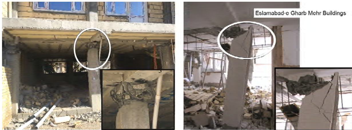
Figure 9. Fracture of a weak story RC column during the earthquake.
