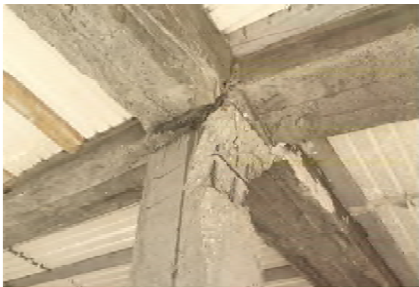
(a) Flexural Damage at the Top of the Column
