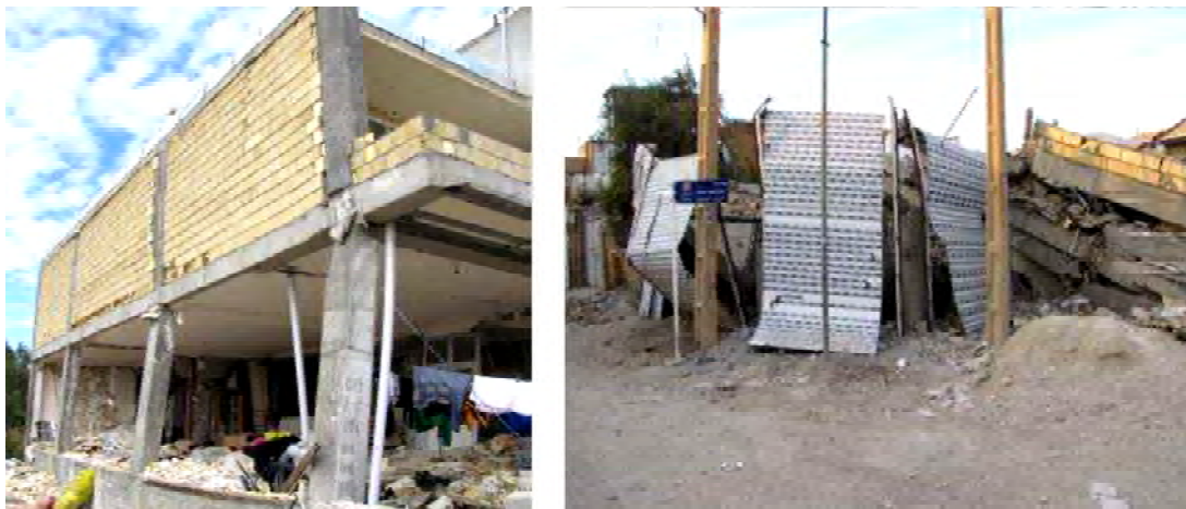
Figure 6. Soft story collapse mechanism in 12 th November 2017, Sarpol-e Zahab earthquake.
