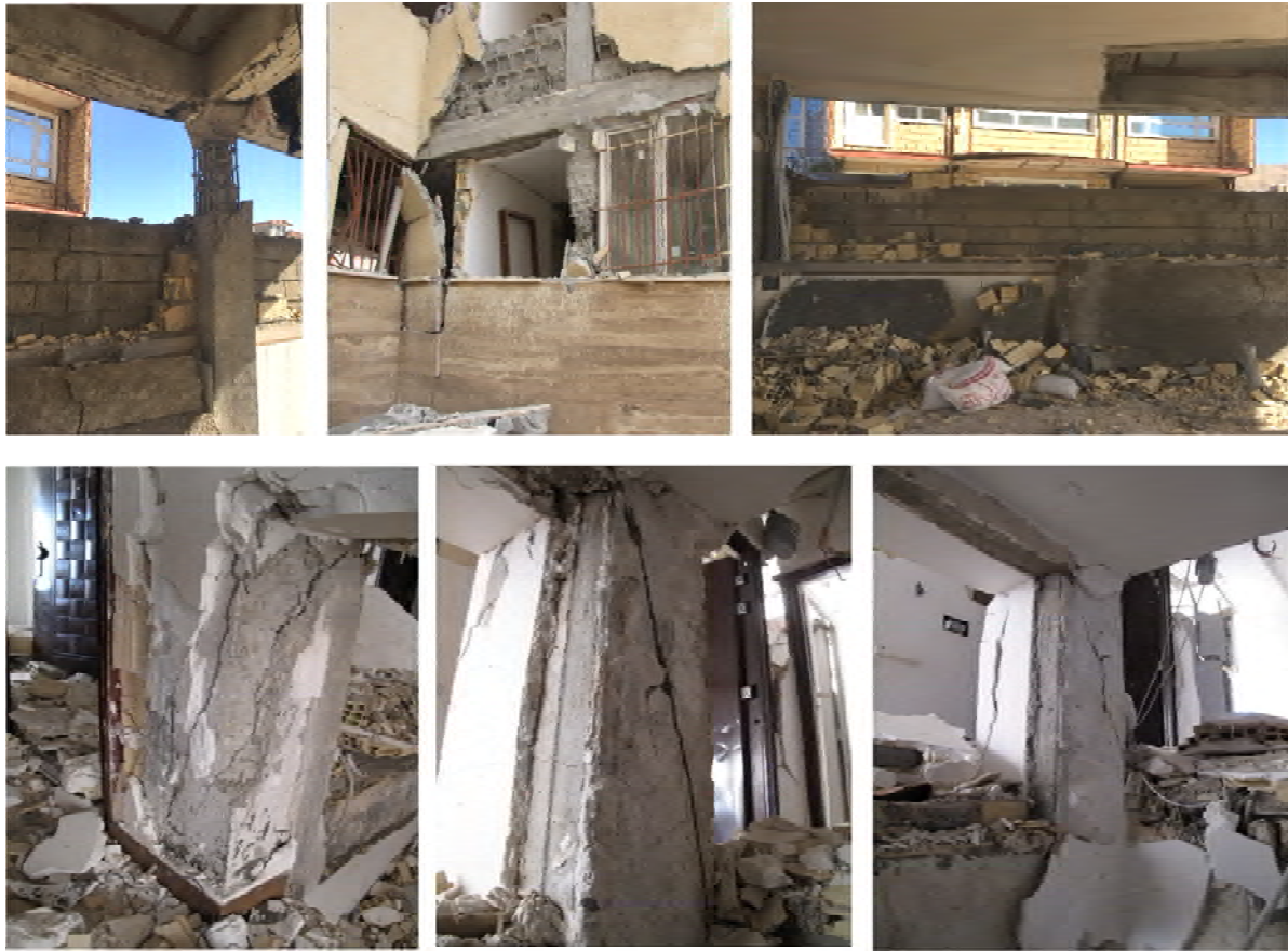
Figure 11. Short column effects in Sarpol-e Zahab, Mehr buildings.
