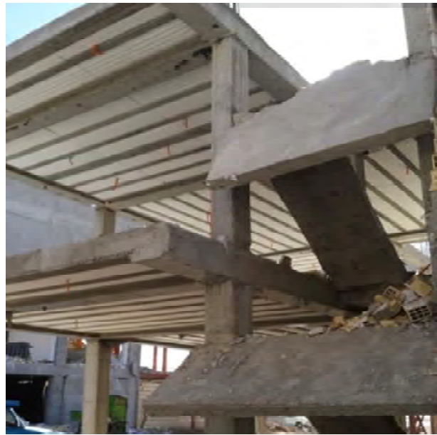
Figure 34. Failure of concrete cantilever slabs of staircase.
