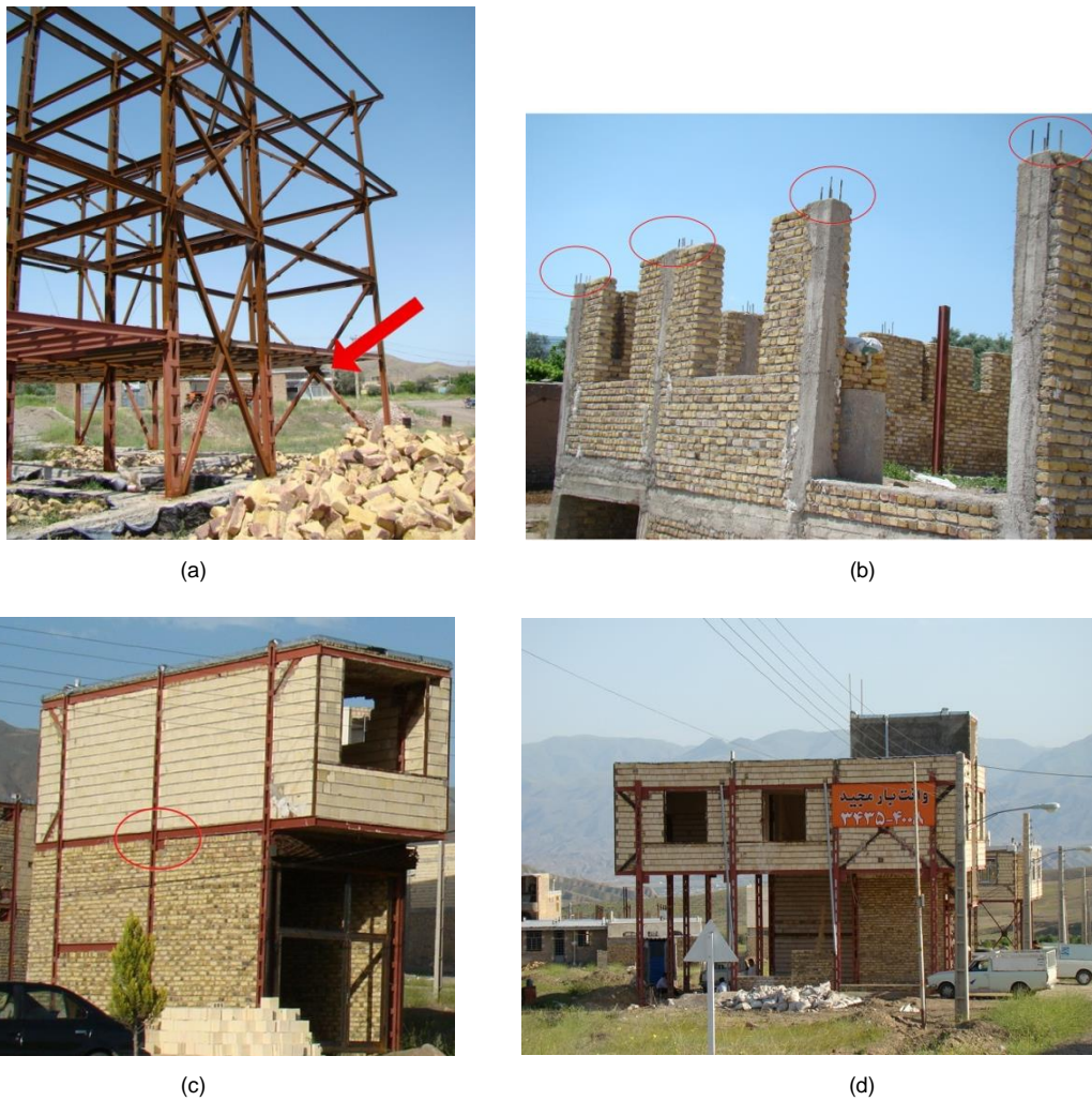
Figure 10. Samples of mistakes in the new and vulnerable constructions: a) An under-construction four-story steel braced structure is shown. The braces did not connect to the first floor so the first floor does not have the lateral load system (shown by arrow in the figure). b) A two-story confined masonry under-construction structure is shown. Inadequate anchorage length of reinforcement in vertical ties has been observed. This creates weak joints in ties and causes damages in an earthquake. c) A two-story steel structure is shown. The gusset plates for braces installed in the columns (shown by circle), but no brace was installed for this building. d) A two-story braced steel structure is shown. The missing braces in the first floor are observed.
