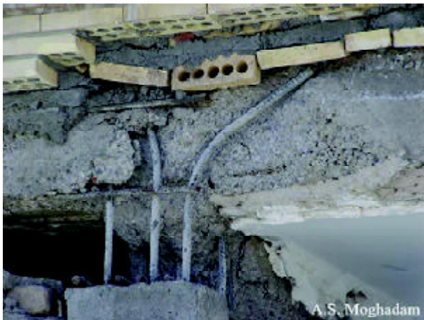
Figure 14. Poor detailing in connection.
