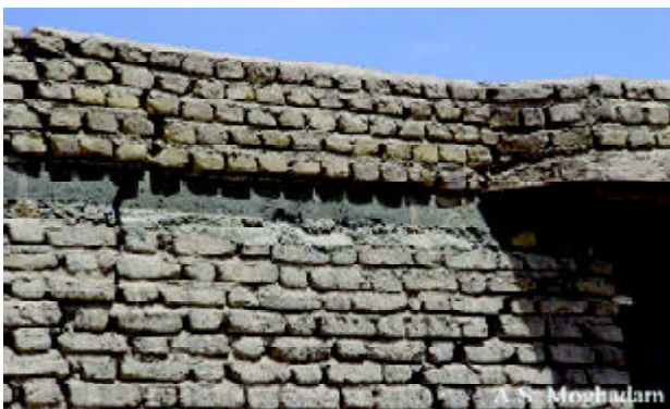
Figure 10. Crack in tie beam due to lack of reinforcement.
