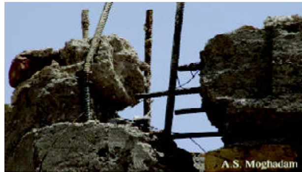
Figure 11. Improper connection of vertical and horizontal tie bars.
