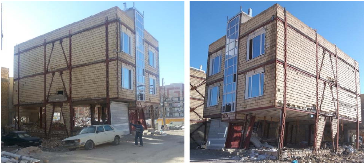
Figure 8. Real view of S-2 building after Sarpol-e Zahab earthquake.
