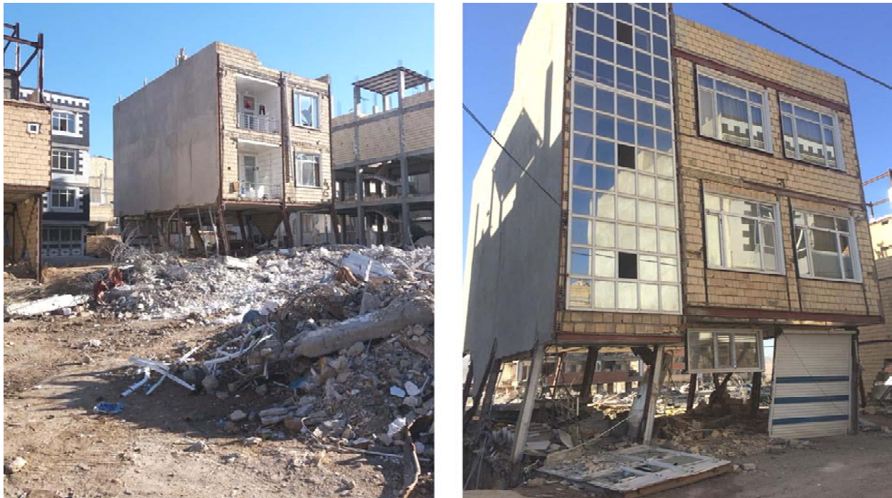
Figure 6. Real view of S-1 building after Sarpol-e Zahab earthquake.
