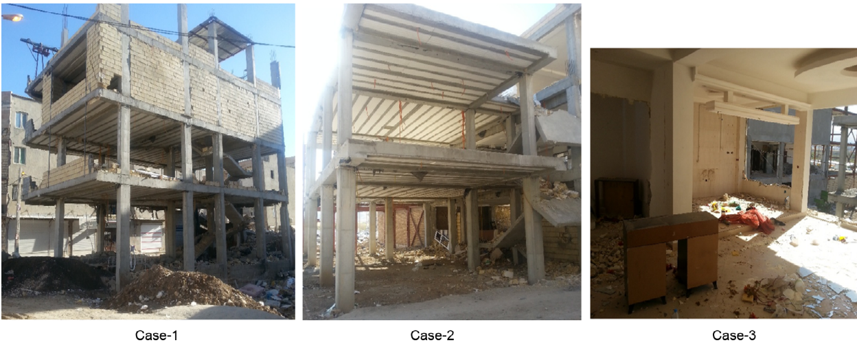
Figure 2. The three heavily damaged buildings after the earthquake.
