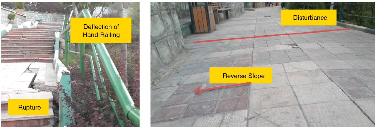
Figure 1. Evidences of slope sliding in the ground surface (static condition).
